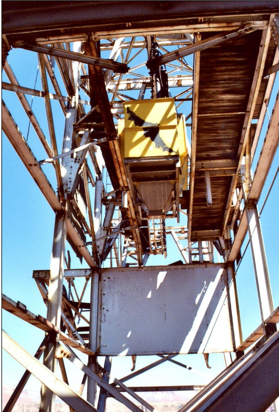
Underside of Bat Cave tram headframe with view of transport car and dump chute on its bottom. View faces toward the canyon. The black-bat livery was painted for the 1959 film, Edge of Eternity .
