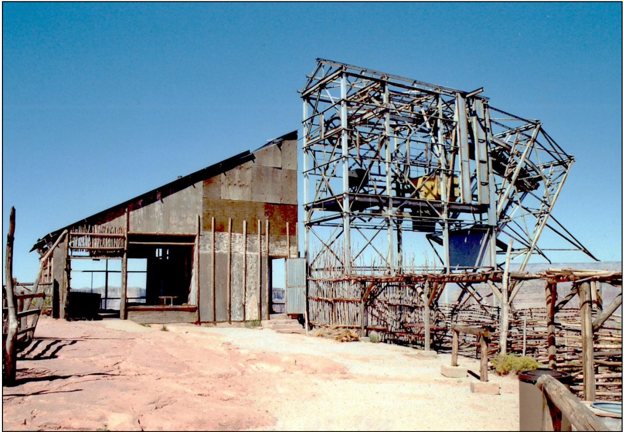
Bat Cave tram headframe. The yellow object is the transport car ( see next page ).
