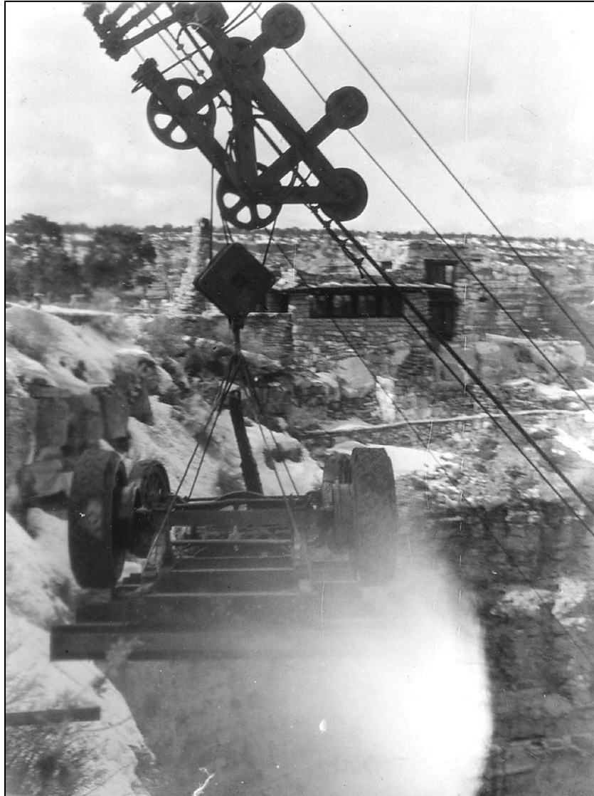
Truck bottom inverted on the Indian Garden tram during water pipeline construction, ca. 1932. (Lookout Studio is in the background.)
